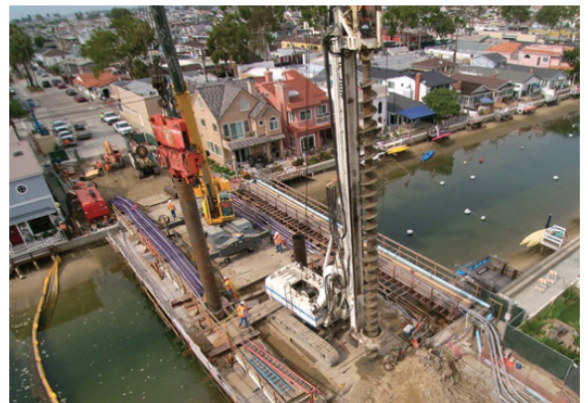
On the Park Avenue Bridge Replacement Project in Newport Beach, California, crews constructed bridge piers and abutments in difficult drilling conditions.
