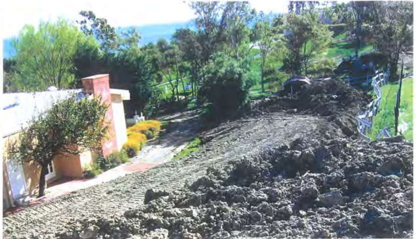
▲ This home in Malibu was saved from a catastrophic landslide during the recent torrential rains on the West Coast thanks to a quick response time from the design team.
